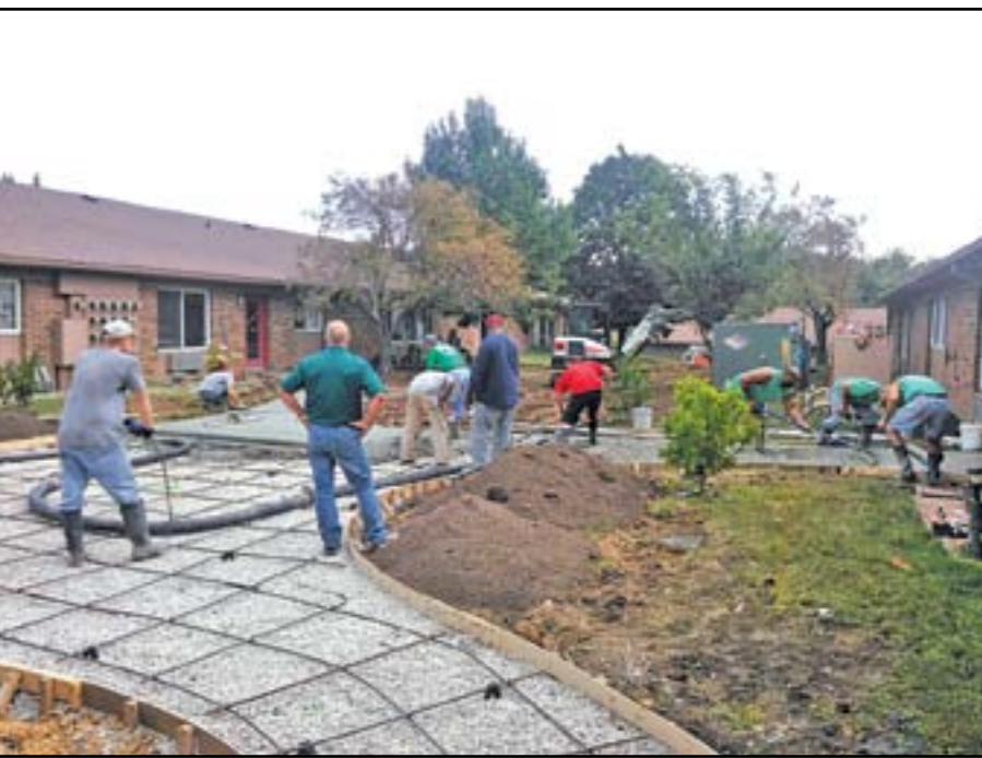
Workers prepare to pour concrete for Orchard Lane Leisure Living's new sidewalks.
