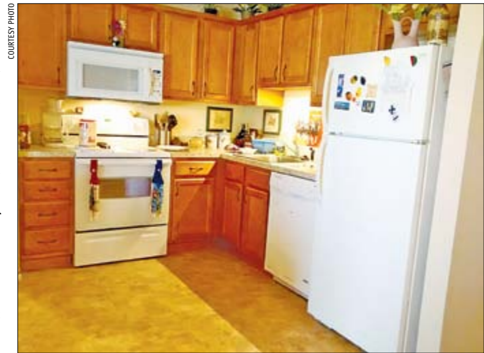
Thanks to an Affordable Housing Program grant, Baldwin City's Orchard Lane Leisure Living is undergoing a major renovation, including new cabinets, appliances, and light and plumbing fixtures.
