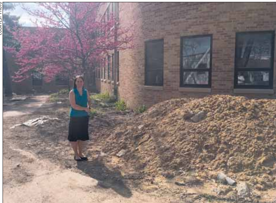
Megan Poindexter at the Senior Resources Center building, which is currently being renovated.
